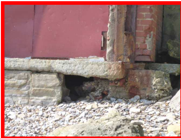
Undermining and voids at disused lifeguard station (/0401C01)
