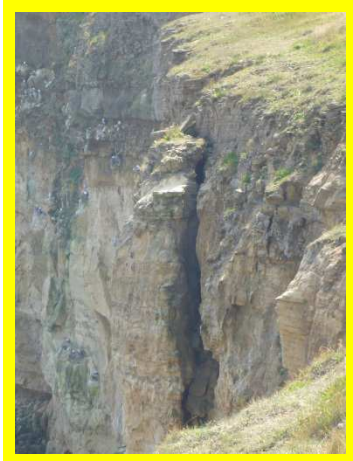
Vertical cracks in the cliff face (/0401C05)
