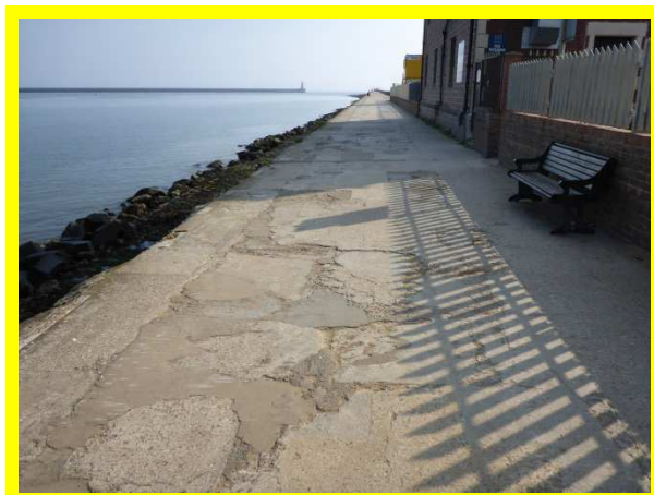
Deck abrasion and previous repairs on South Pier (/0103C01)
