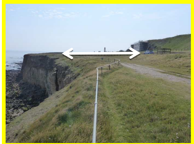
Proximity of cracked cliff to Coast Road (/0401C05)
