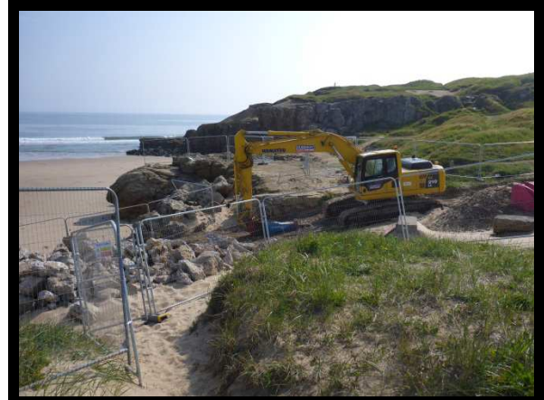
Old slipway demolished ready for construction of replacement at southern end of Herd Sands (/0202C01)
