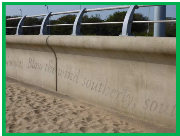
Central section of Littlehaven promenade and seawall in very good condition (/0102C02)
