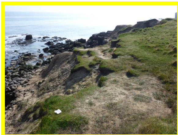
Localised slumps in soft material at Trow Point Trow Point (/0302C01)
