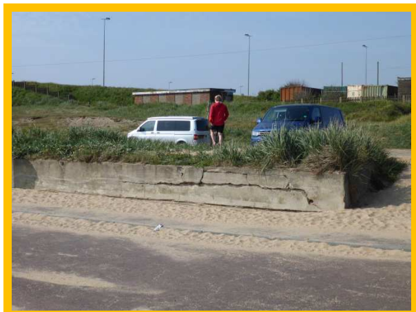
Cracking in wall to rear of promenade at southern end of Sandhaven (/0202C01)
