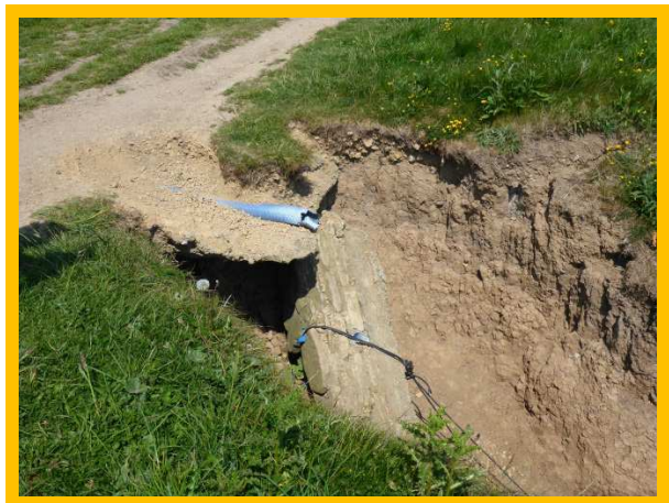
Failed headwall due to localised slumping (/0601C02)
