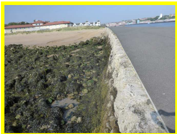
More sheltered southern side of South Groyne in fair overall condition (/0101C02)
