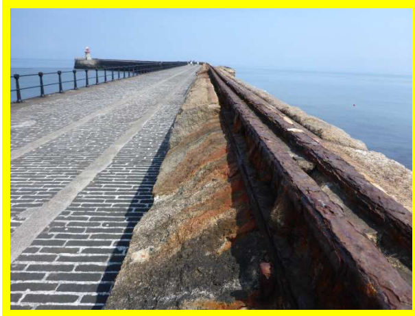
Deck abrasion/spalling and previous repairs on South Pier (/0103C01)
