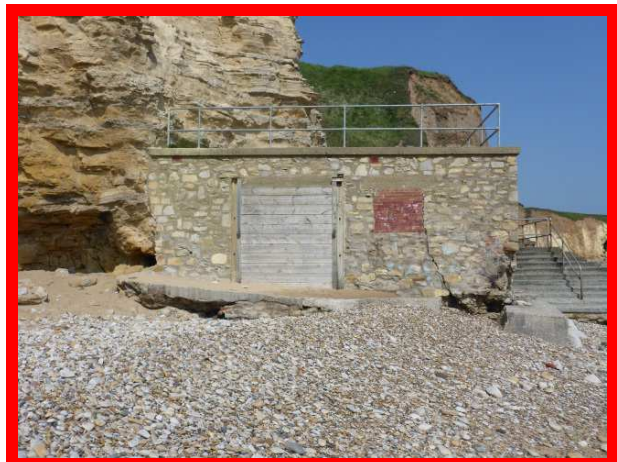
Undermining and cracking at storage building on south face of buttress to access steps (/0401C01)
