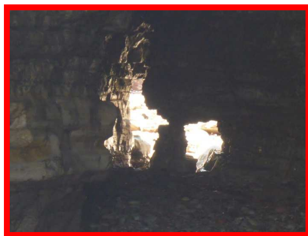
Enlarged cave hole at the former Old Harbour Quarry – detailed view (/0501C01)
