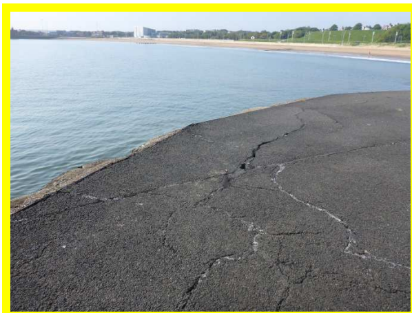
Localised cracking in bitmac deck at seaward end of South Groyne (/0101C02)
