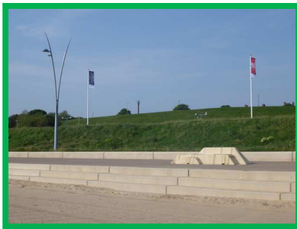
Northern section of Littlehaven promenade and seawall in very good condition (/0102C02)
