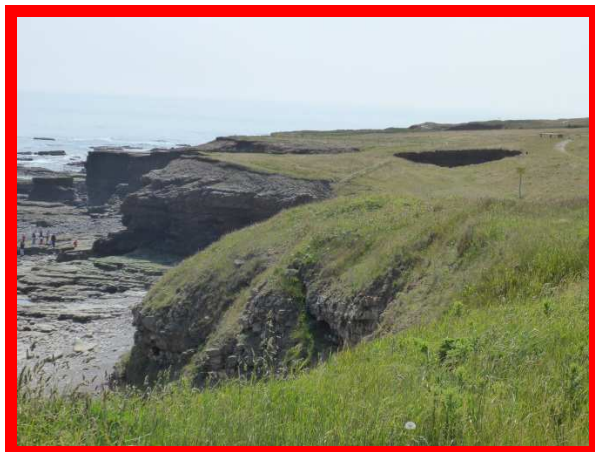
Enlarged sink hole at the former Old Harbour Quarry – general view (/0501C01)
